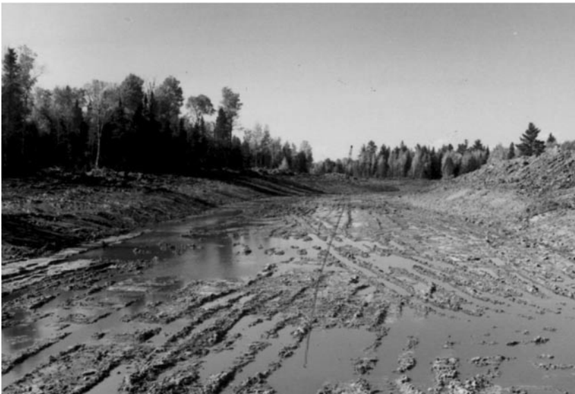
FIGURE 8. Nett Lake River channel after improvement, the width is 80 feet. Photo courtesy of the MNDNR.
